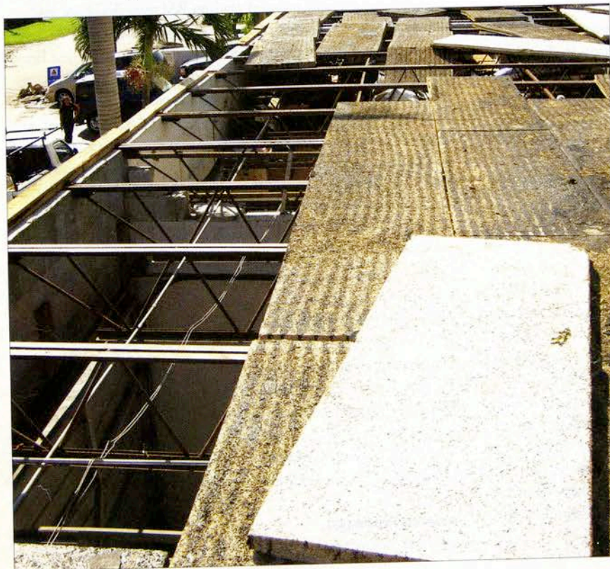
Many commercial buildings were damaged when roofs peeled back, revealing metal decking, such as this roof in Pompano Beach, FL. (Photo courtesy of Billy Cone, president, Rooftech Roofing & Sheet Metal, Ft. Lauderdale, FL.)
